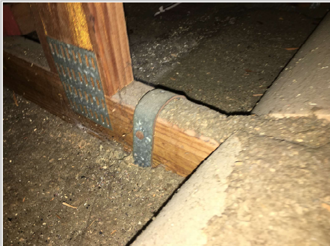
Toe Nail - Straps not meeting nail requirements
